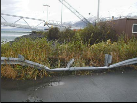
Damaged Railing at East Approach Ramp
