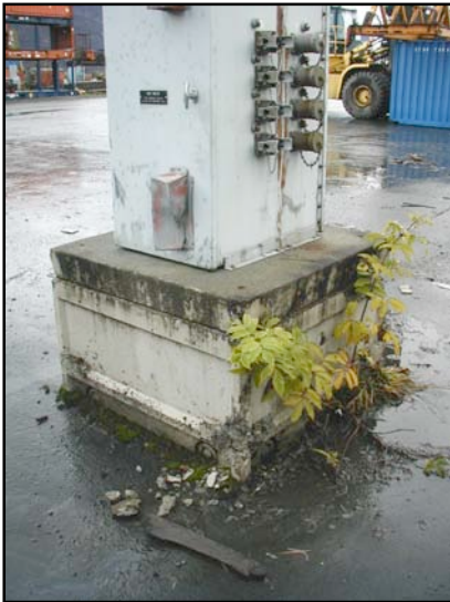
Damaged Power Pedestal
